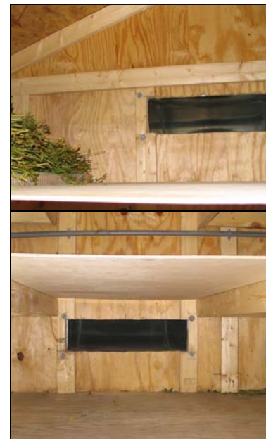
Figure 11: Upper and lower vents. These are the two points where the ductwork connects to the rear of the building. Air circulates into the shed via the lower vent, and back through the heating ducts via the upper vent.
