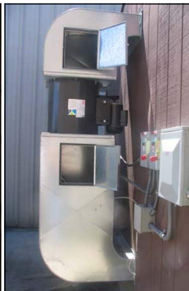
Figure 9: Duct work and access doors housing heating elements and fan
