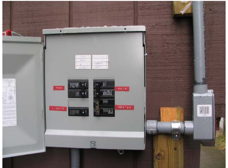
Figure 13: Fuse box with different switches for fan, heat, light, and main.
