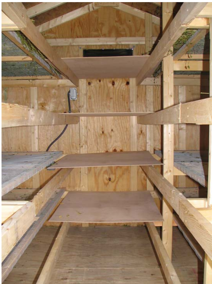
Figure 10: The interior of a modified utility building. Note the four levels of shelves on either side of the center aisle. Plywood spacers span the aisle to direct airflow up through the material on either sides of the aisle.
