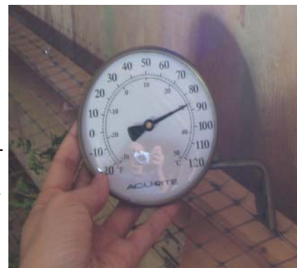
Figure 3: 120°F Thermometer mounted inside the drying unit..
