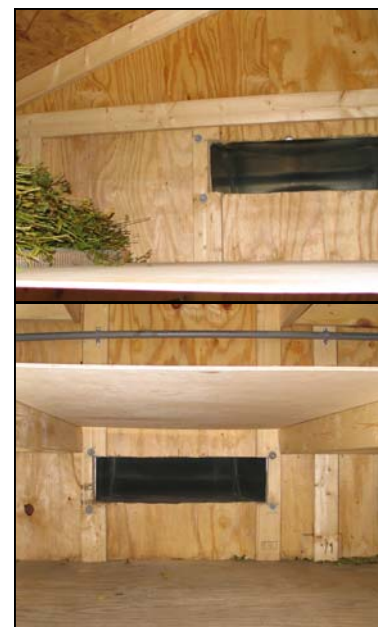
Figure 11: Upper and lower vents. These are the two points where the ductwork connects to the rear of the building. Air circulates into the shed via the lower vent, and back through the heating ducts via the upper vent.
